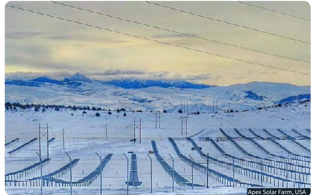
Apex Solar Farm, USA
